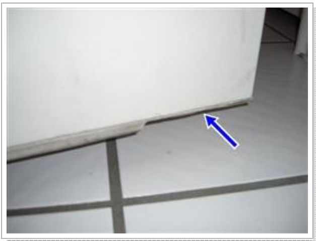
Damaged threshold seal noted at base of laundry room to garage door.
