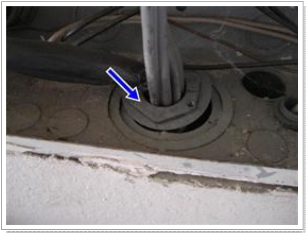
Missing panel bushings at added wiring in main panel.
