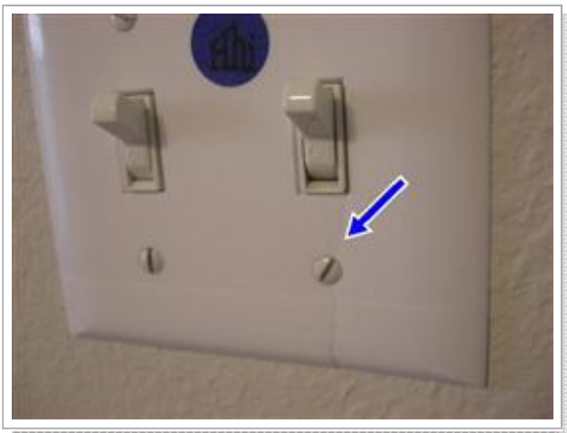
Damaged/ cracked receptacle cover noted in bedroom. Marked with blue dot.
